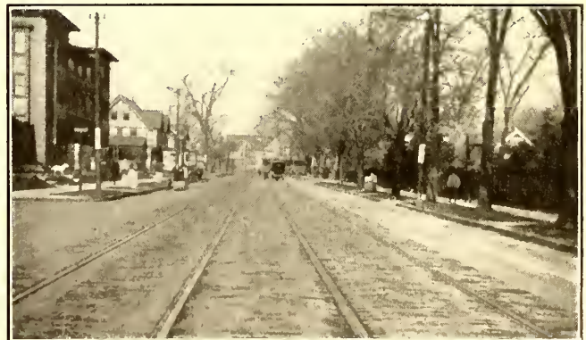
CONDITION OF TRACK AND PAVEMENT THREE YEARS AFTER RAILS WERE REPLACED BY AID OF OAK SHIMS
